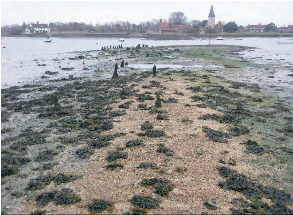
Fig 14 This failed seawall was constructed across Bosham channel in the early 19th century (CHC0059, Maritime Archaeology Ltd 2006a)
